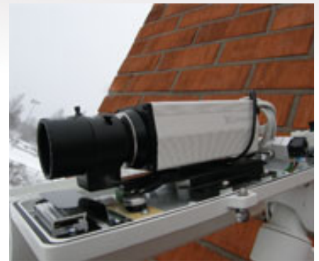
Avalarm Surveillance Installation Featuring Lumenera's Le175 Digital Camera
